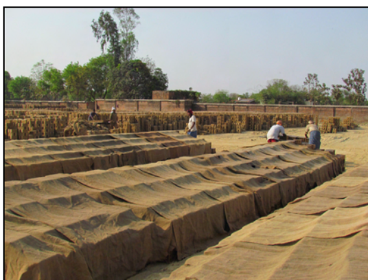
Figure 3.6: Hacks are covered with sheets to prevent cracking during adverse weather conditions
