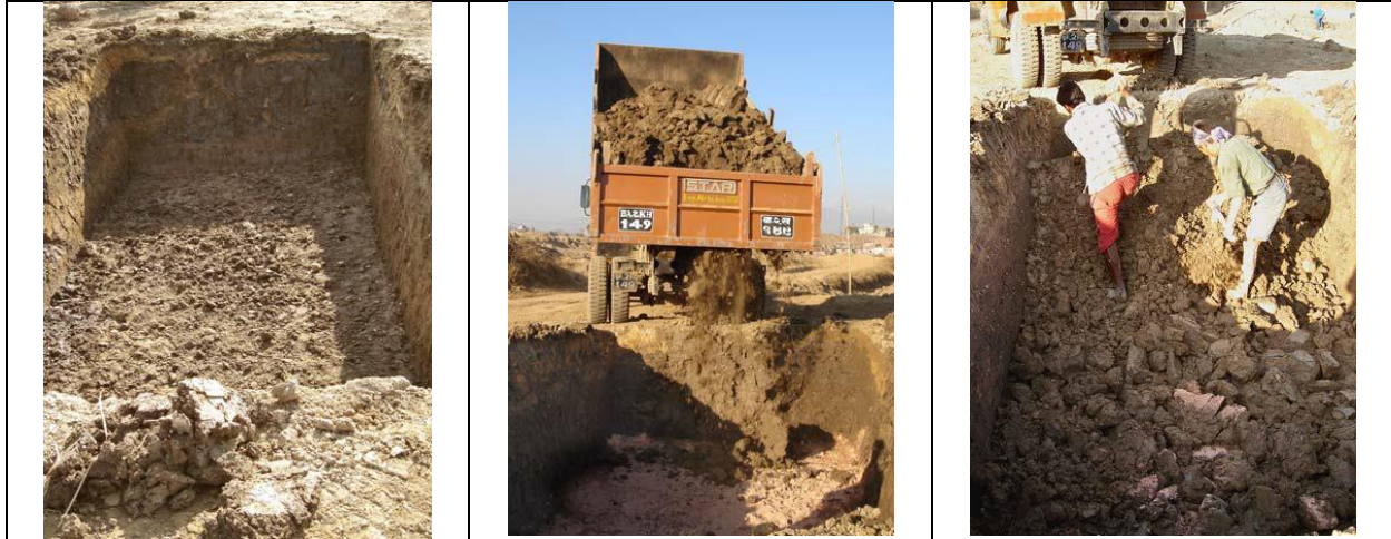
Figure 40: Soil preparation tank 17
