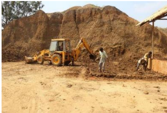
Figure 15: Raw mix preparation area
