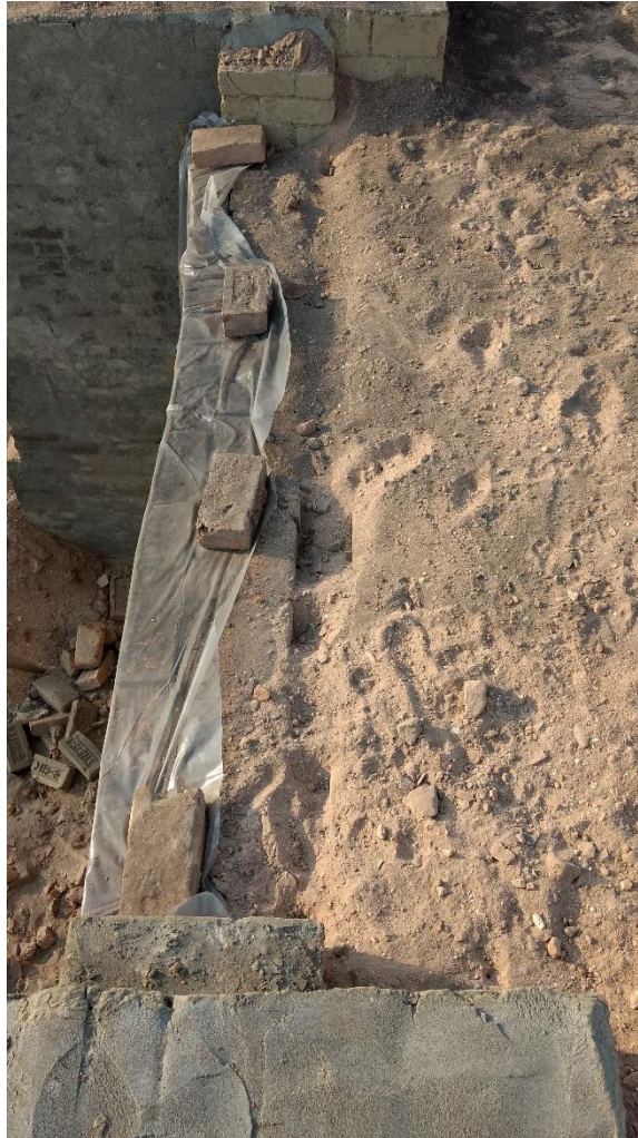
Figure 97: Proper closing of wicket during firing
