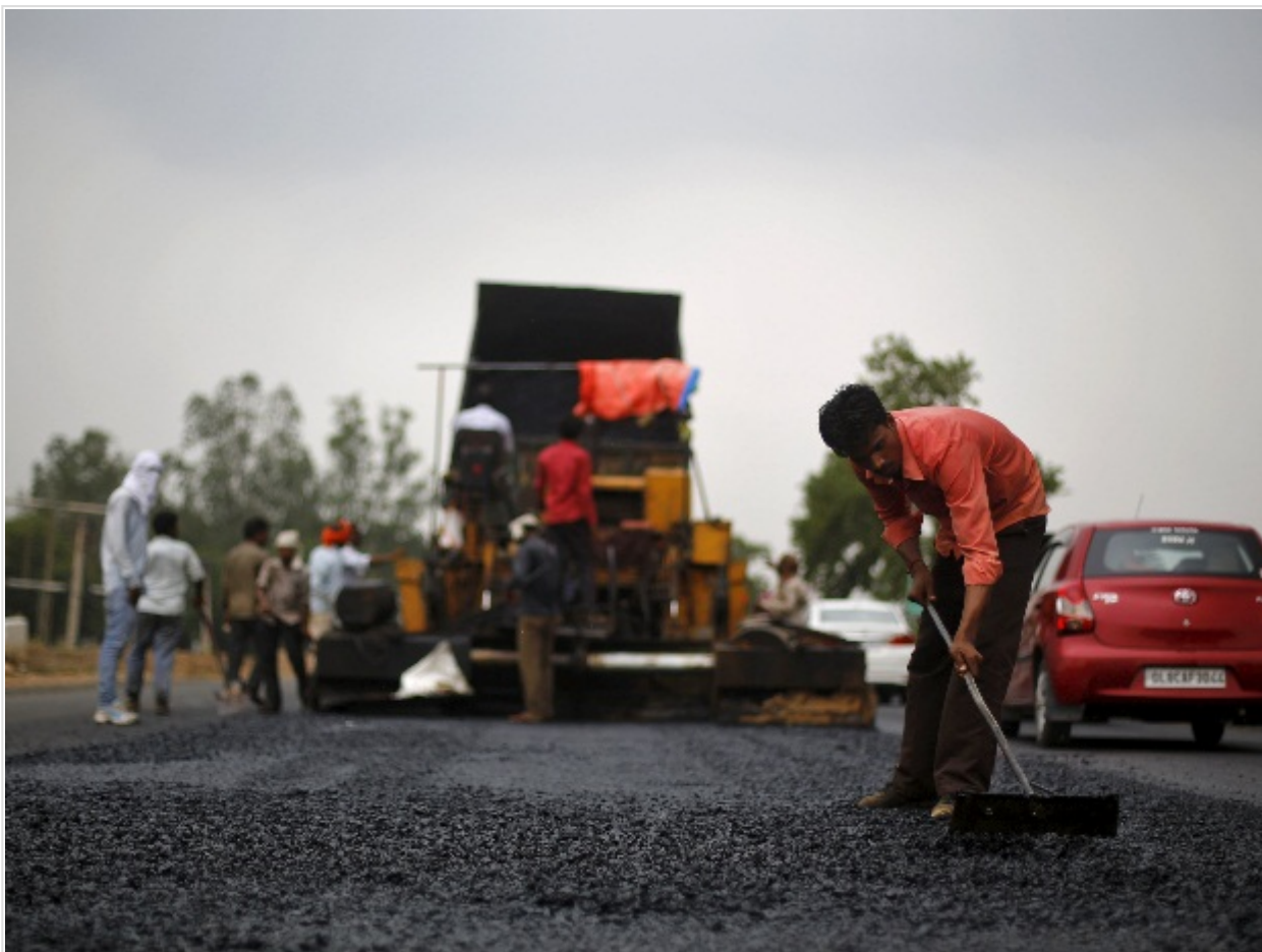
labourer works at the construction site of the Delhi-Jaipur national highway in Manesar in Haryana
